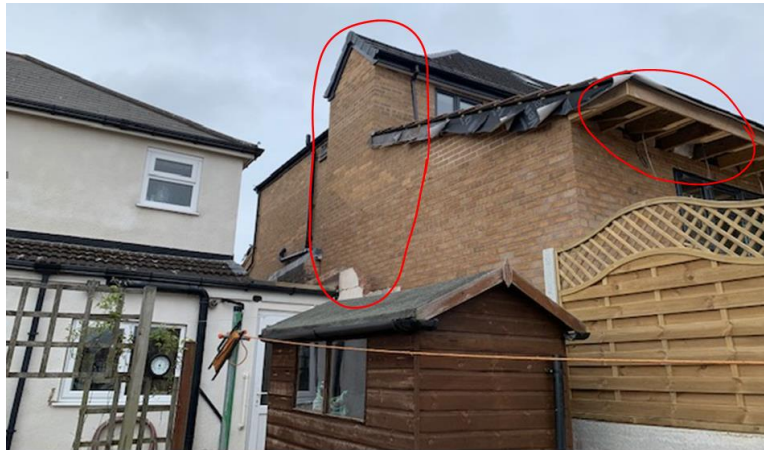
Fig 3: View from the rear garden of number 78. The unauthorised elements are circled (first floor extension and rear canopy).
